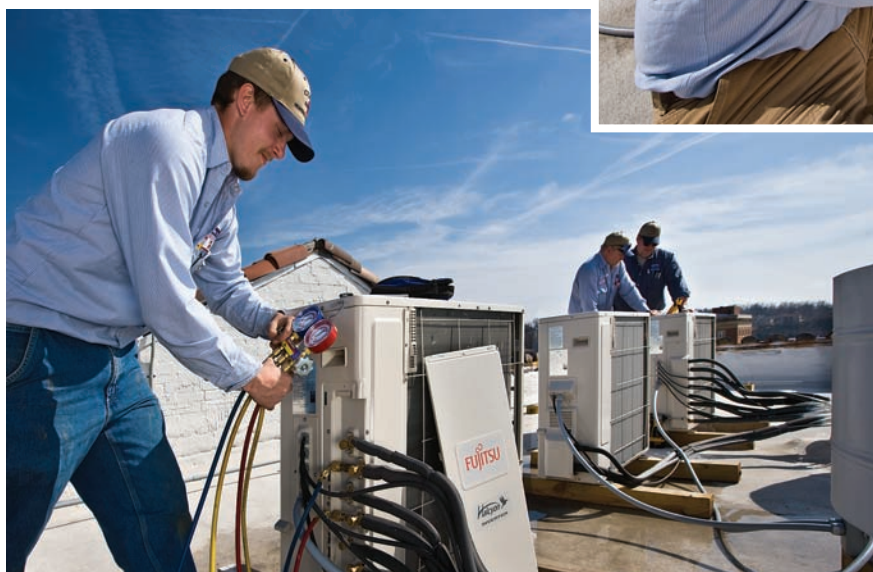
Cash Curtis, service technician, checking R410A refrigerant charge. In the background, David Conner, service manager, and service tech Philip Curtis, owner, checking proper voltage and operation.
