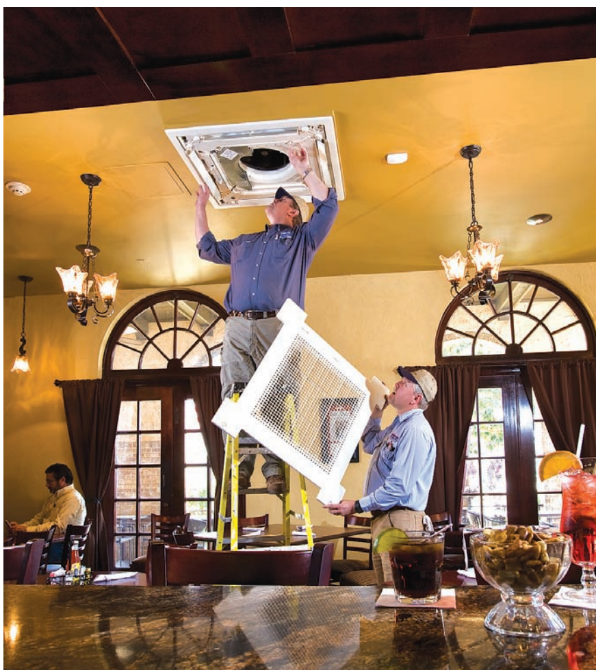
Philip Curtis, owner, on ladder, with David Conner, service manager and tech, in the Hotel's restaurant installing an air intake grill and cover on a ceiling unit.
