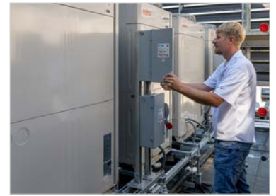
Darnold Mechanical's Spencer Faber inspects the disconnect on an Airstage condenser during commissioning.
