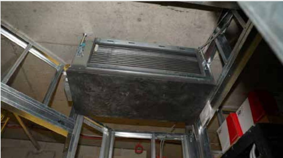
A three-ton air handler is used to condition the office and locker space behind the bar.
