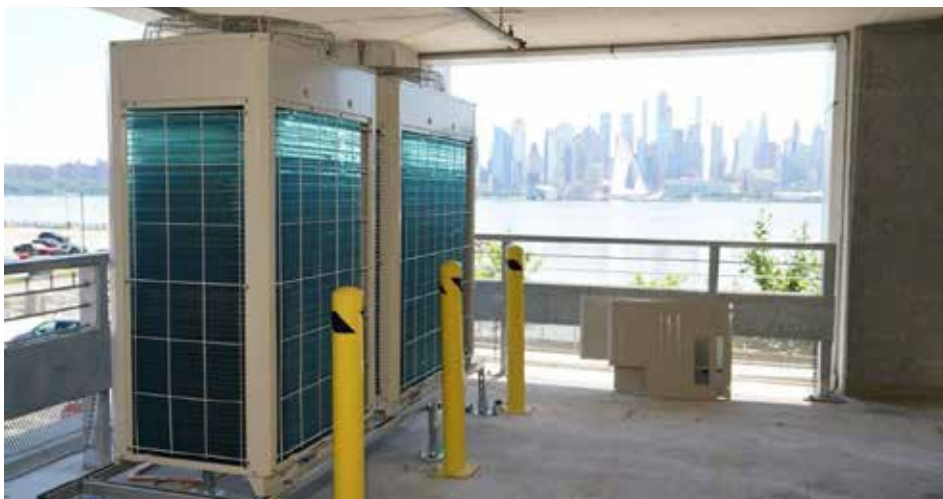
Because the restaurant is in the lower level of a parking garage, there were very few options when it came to placing the VRF condensers.
