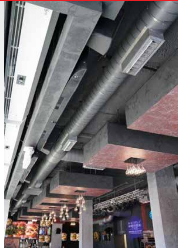
Large, high static air handlers are used to heat and cool the seating area through exposed spiral duct
